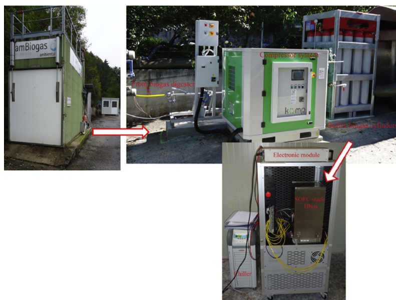
Fig. 6. Complete pilot plant for the energy generation with SOFC built.
